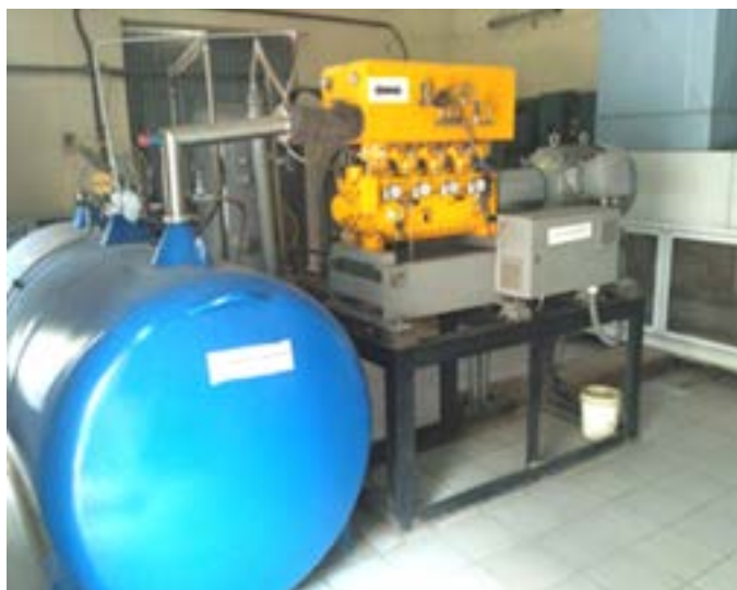
Liquid Nitrogen Plant
