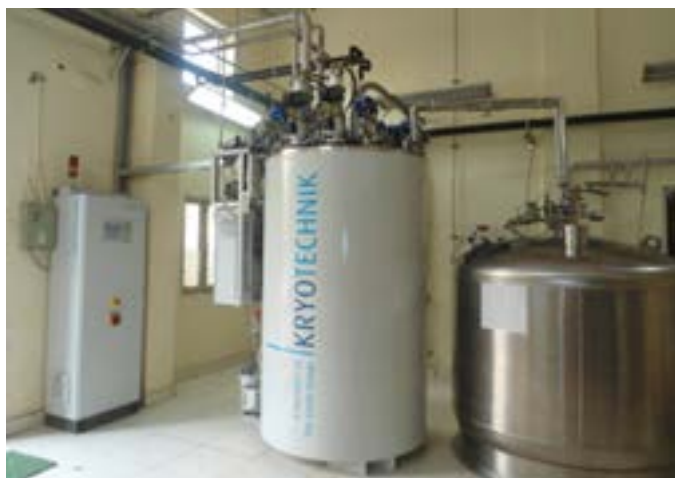
Liquid Helium Plant
